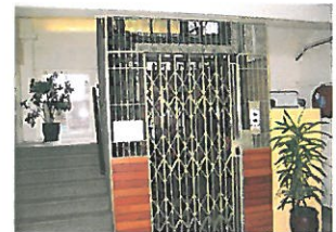
Fully functioning cage elevator, shown here on the ground floor
